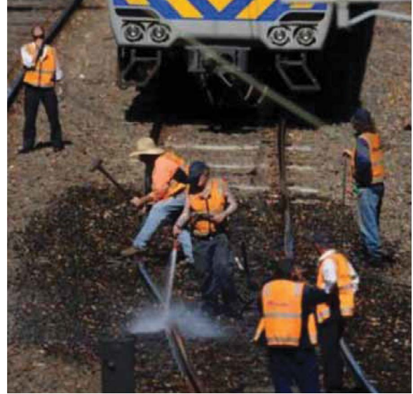
Figure 7: Rail tracks in Melbourne buckled during the 2009 heatwave.
